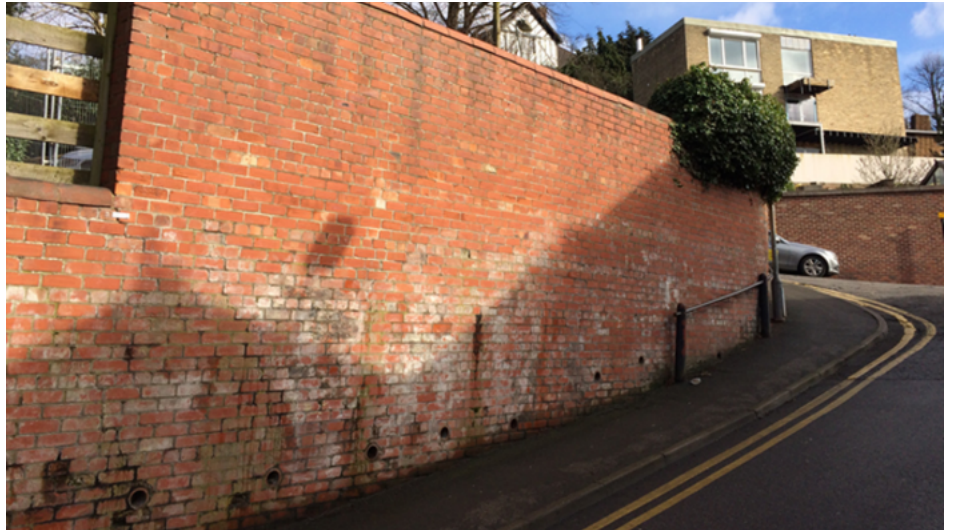
The unsafe wall at Beaumont Lee
